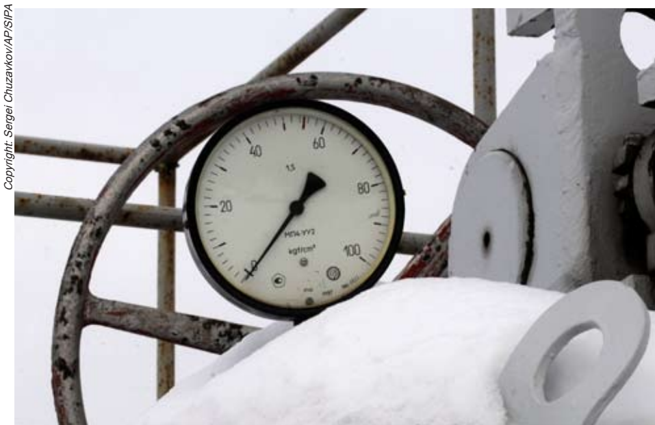
A gas pressure gauge indicating zero on the main pipeline from Russia near Kiev, January 3, 2009.
